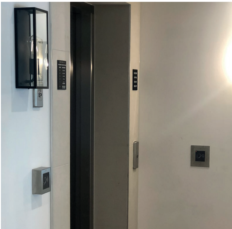
Lift calling is also proximity reader controlled.
